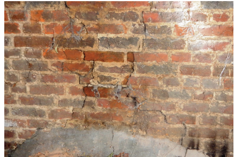
Barsten in stookmuur schoorsteen.
